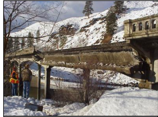
The sidewalk fell off of Bridge 153/20 in 2002.
